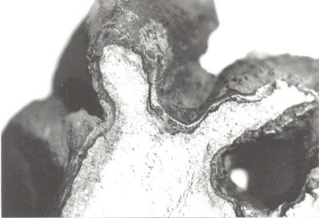
F 3 This fractured surface demonstrates clearly a 1 mm thick pollution / gypsum crust on the limestone surface
