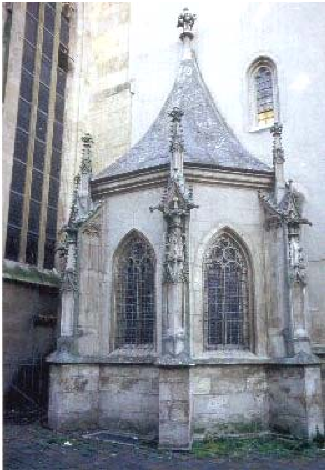
F 1 Cathedral Eichstätt / choir of the capital sacristy Stone surfaces intensely polluted and encrusted Upper areas, especially roofage is overgrown with green algae and moss. Condition before the cleaning
